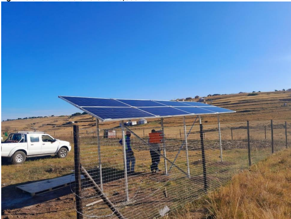
Fig. 2 Installed Solar Panels
