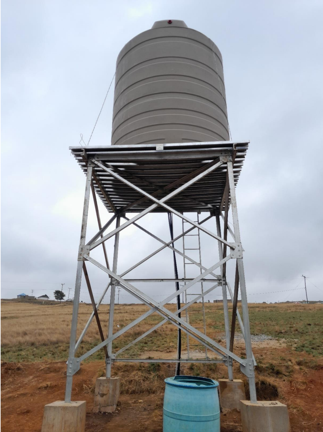
Fig1. Installed Tank stand and 10,000L Tank
