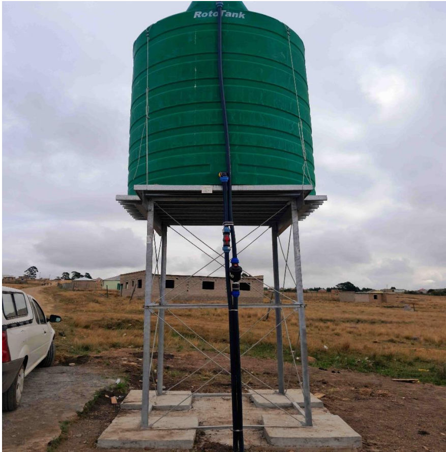
Fig1. Installed Tank stand and 10,000L Tank
