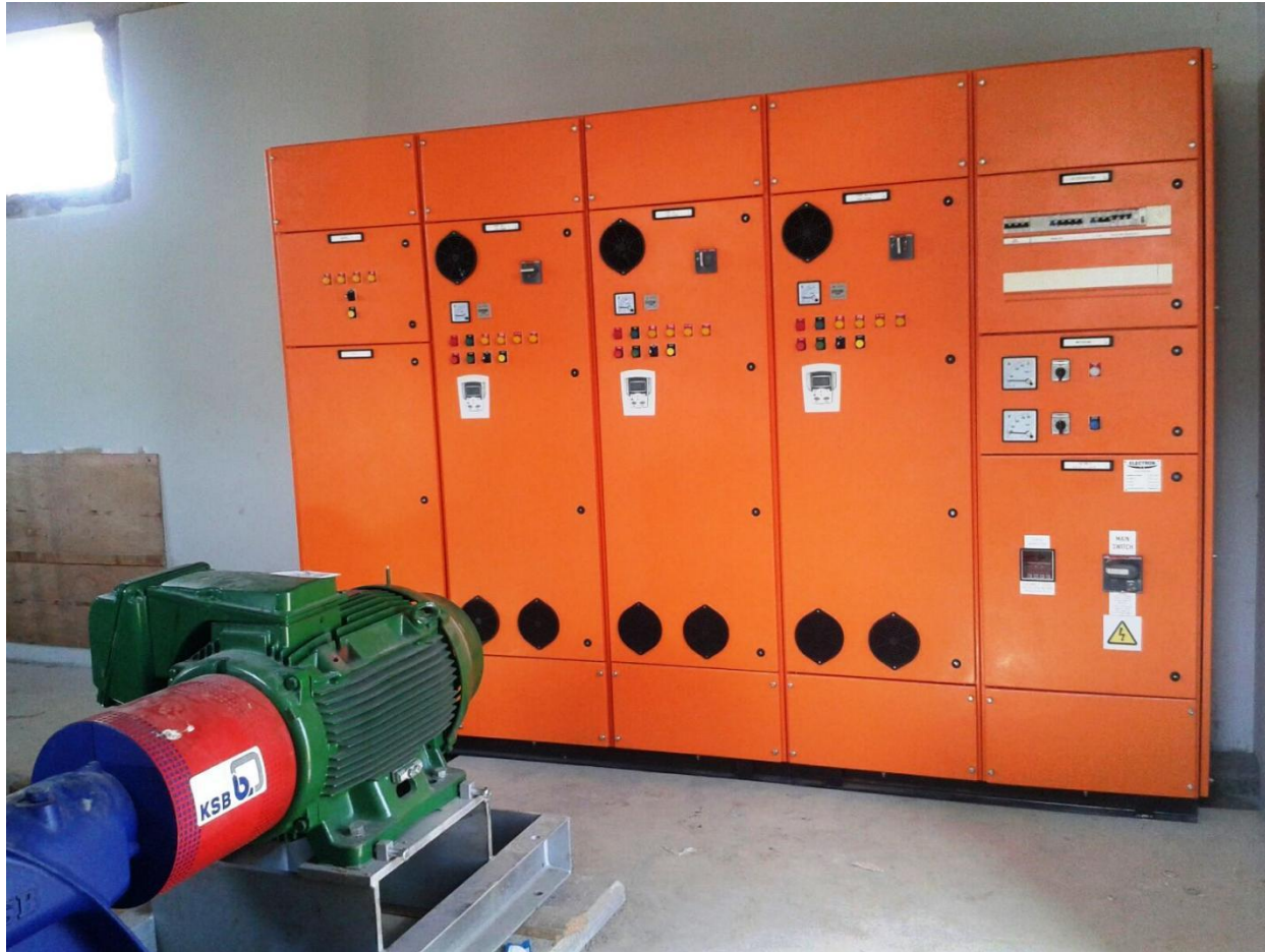
Treated Water Pumpstation MCC
