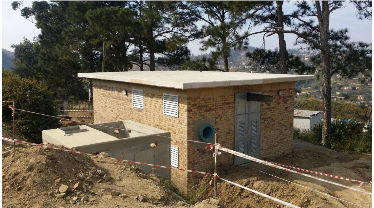
Treated Water pumpstation
