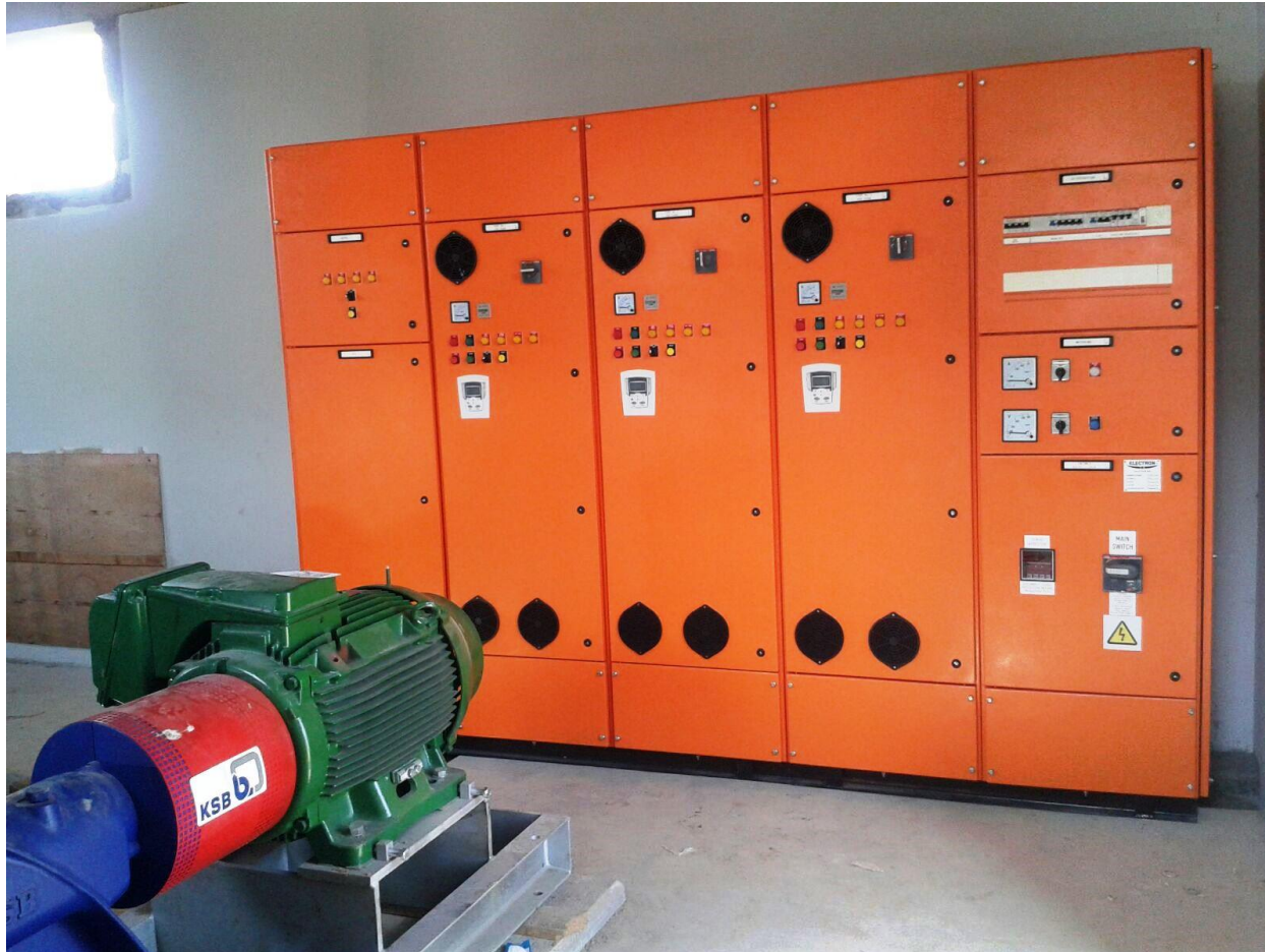
Treated Water Pumpstation MCC
