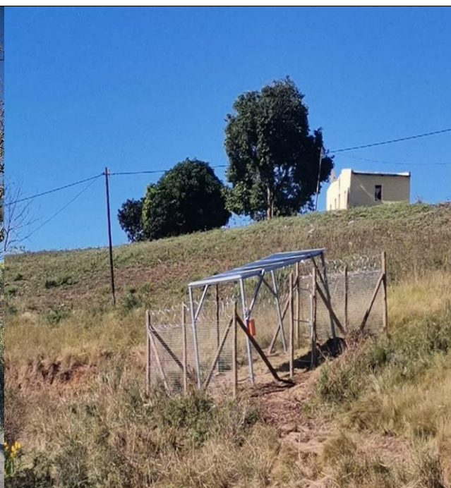
Solar Panels for completed borehole: Sunduza Ray Nkonyeni Municipality Ward 29
