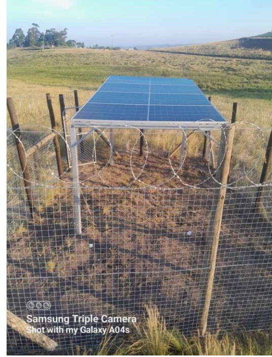
Solar Panels for a completed borehole : Amahwaqa Mzumbe Municipality Ward 11
