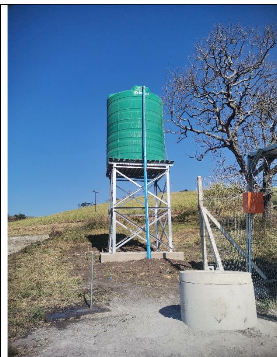
Tank stand, Standpipe & Related Pipework: Rossimin 2 Ray Nkonyeni Municipality Ward 14
