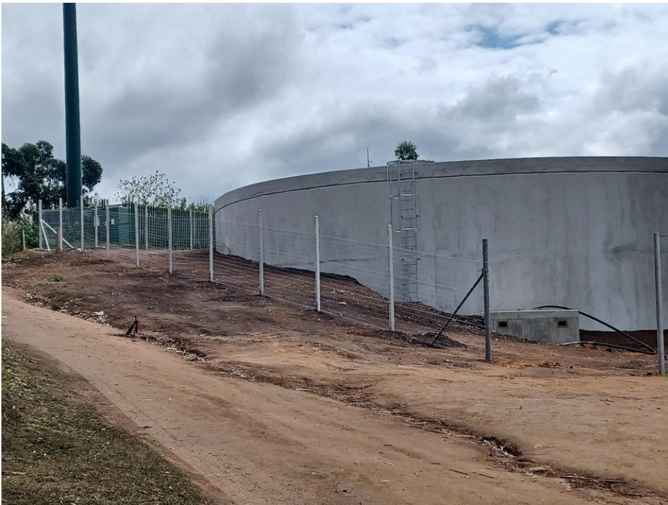
Complete 2ML Concrete Reservoir
