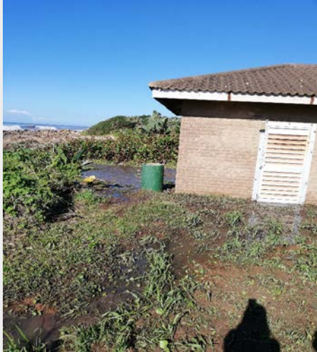
Picture 4 - Discharge from pump house resulting in sewer overflow
