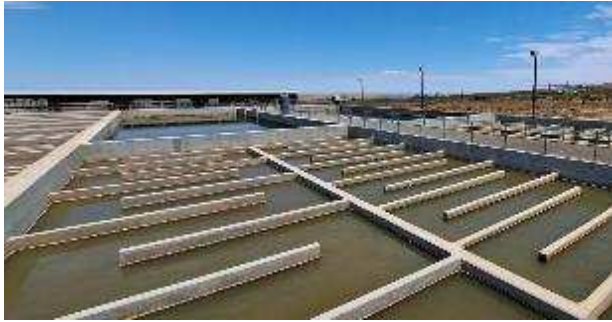
Flocculation channels at Withoogte WTP
