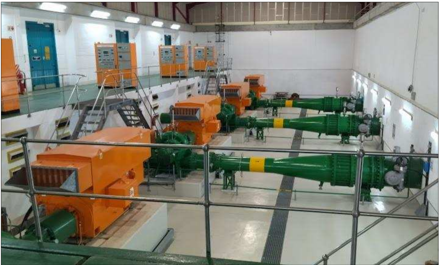
Firlands raw water pump station in excellent condition
