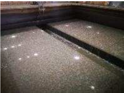
Filter backwashing at Vereeniging WTW
