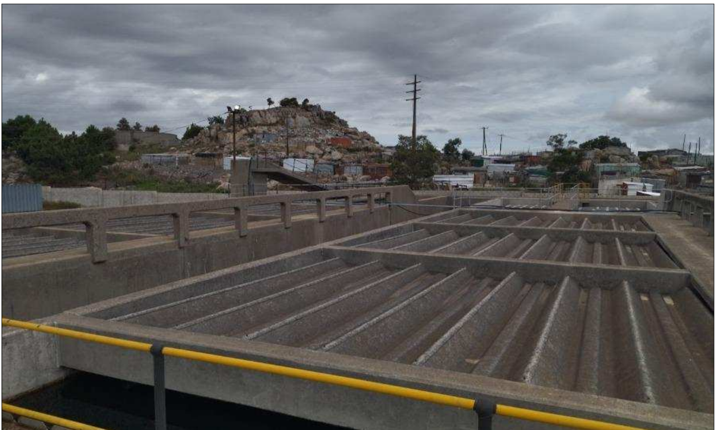
Theewaterskloof: Grabouw WTW clarifiers, routine monitoring to ensure optimal clarification
