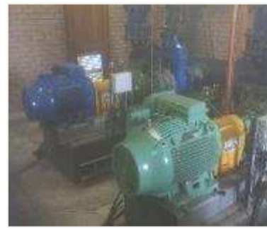
Pumps to the command reservoir
