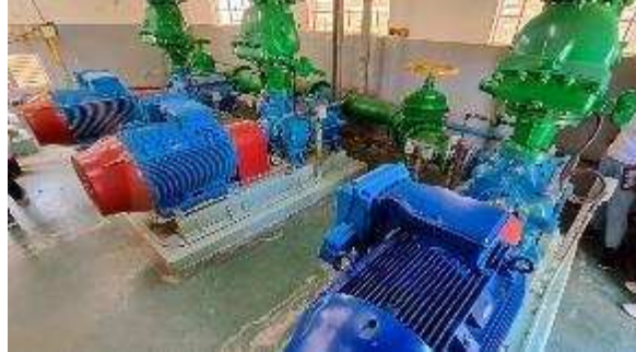
High lift Pumps at Ruensveld West WTP
