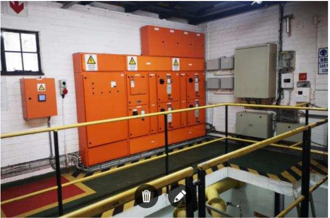
City of Johannesburg and Rand Water: Clean and well maintained pumpstation at Illovo Reservoir
