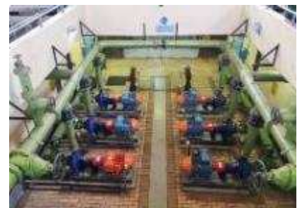
Six recycle pumps are installed and are new and in good condition
