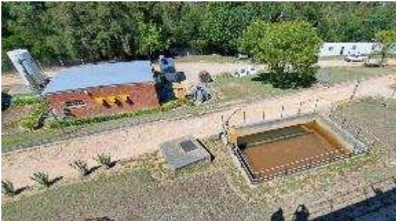
Backwash water sump next to the high lift pumpstation
