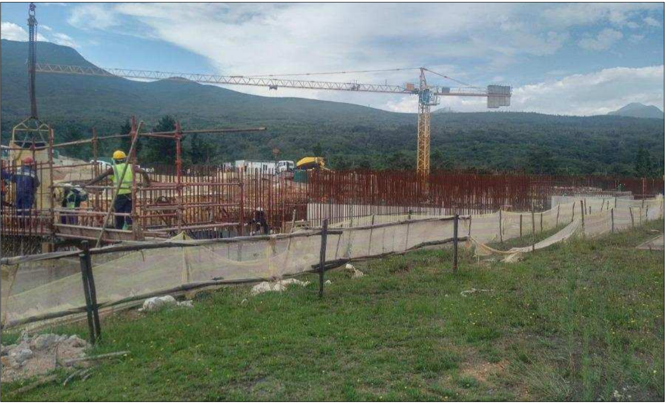
George WTW: Construction underway to expand the water treatment capacity to meet the growing demand
