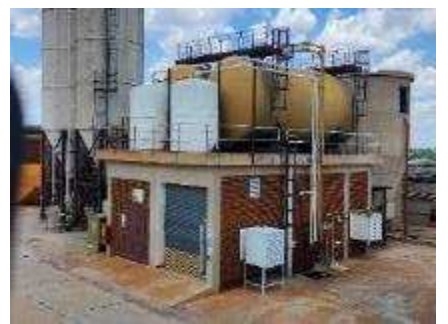
Bulk chemical storage at Balkfontein WTW
