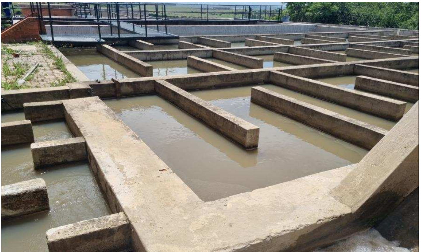
Vaal Marina WTW: daily operational monitoring to ensure high quality water
