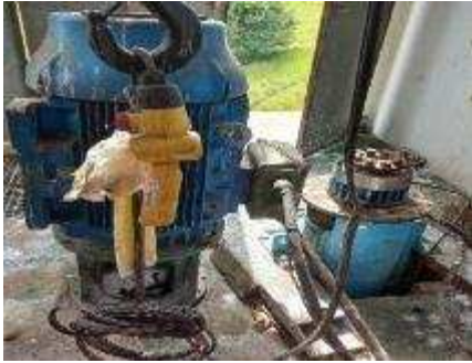
Ngagane river pump station
