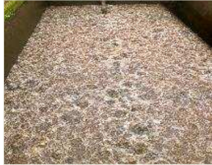
Filter renovation required at Ebenhezer and Doorndraai water treatment plants
