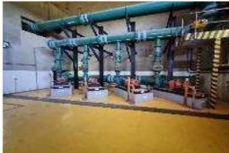
Backwash pumps at Midmar WTW
