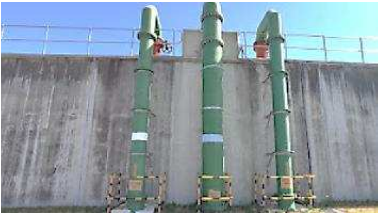
City of Cape Town: Mixing chamber receives softened influent, bypass and water from Melkbos.
