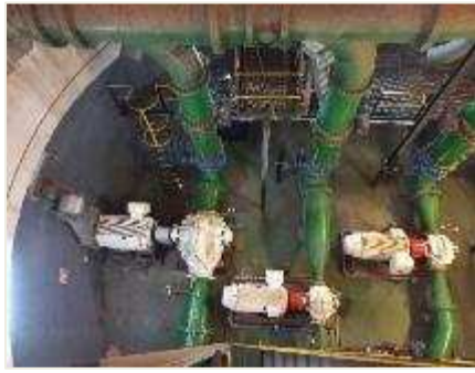
Well maintained raw water pumpstation
