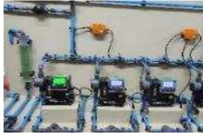
Excellent chemical dosing system at Bethulie WTW
