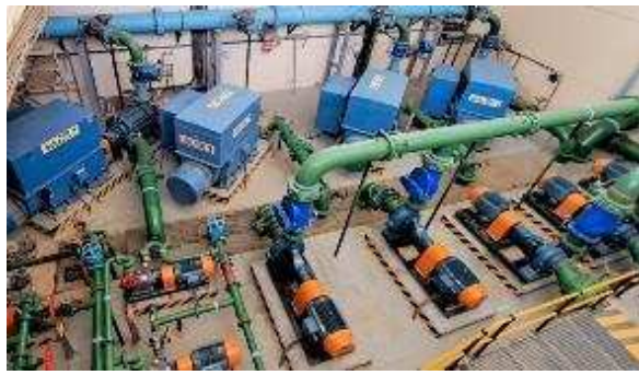
Service and High Lift Pumpstation at Swartland WTP
