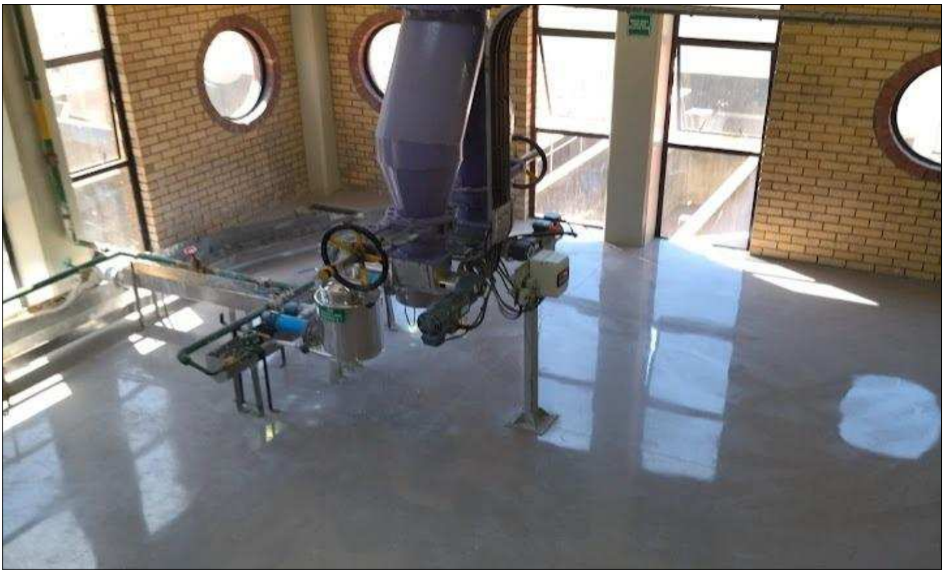
City of Cape Town: Faure WTW lime dosing in prime condition, exemplary of a clean well operated plant
