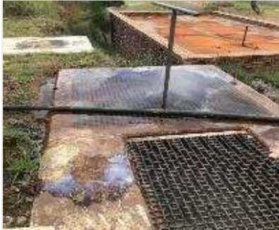
An example of infrastructure maintenance failure at Doorndraai plant contributing to water losses
