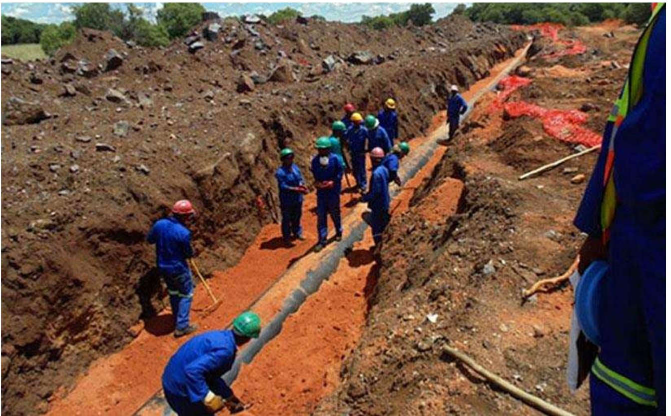
Rand Water: Upgrading of bulk water pipelines to meet current and future demand ( open source )
