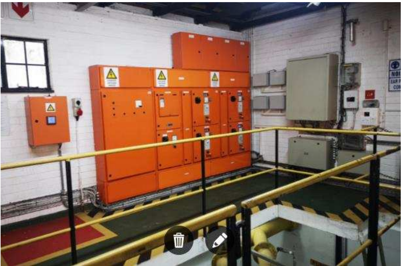
Witzenberg WTW: Pumpstation and motor control centre in mint condition
