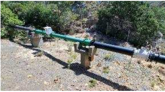
Raw water pipe at Ruensveld West WTP
