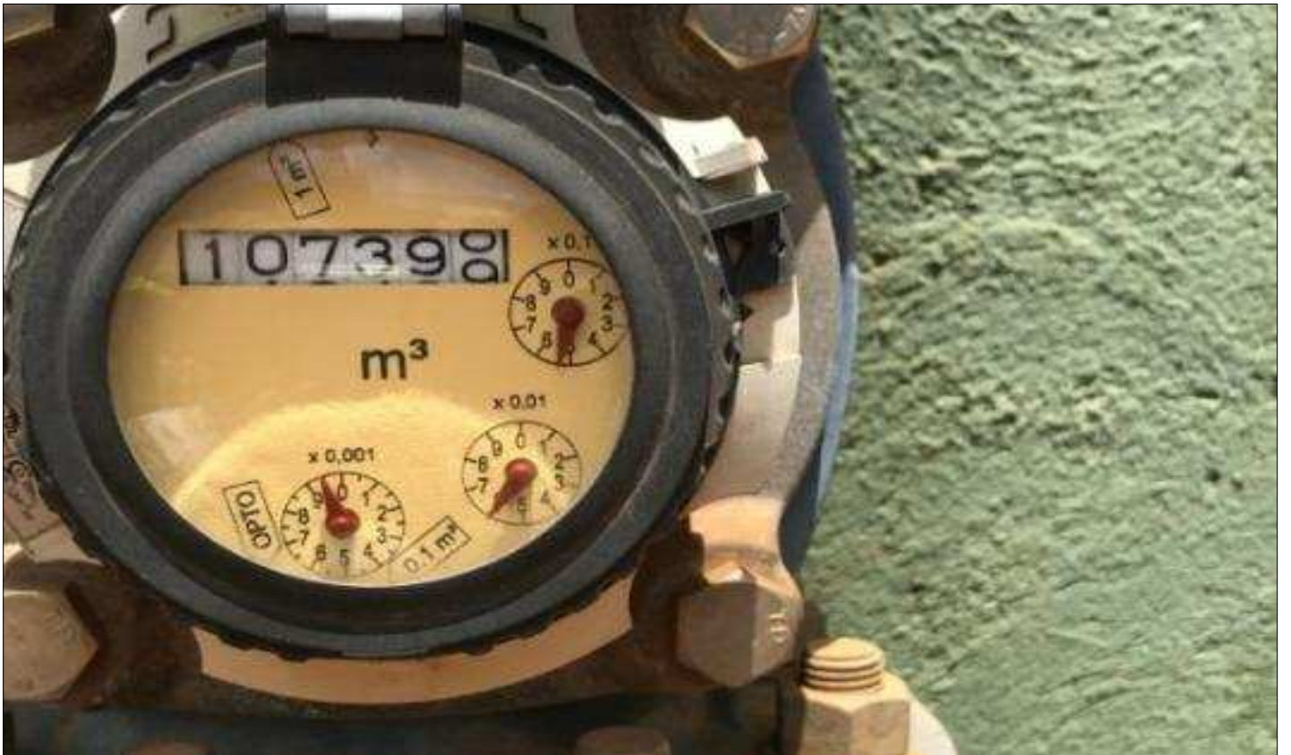
Mbombela/Umjindi: WRCW WTW raw water meter read daily, calibrated
