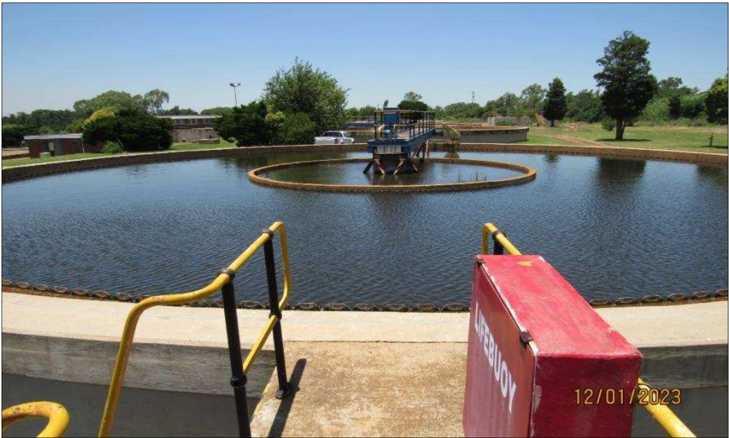
JB Marks: Settling tanks in immaculate condition, cleared of solids, delivering SANS241 compliant water
