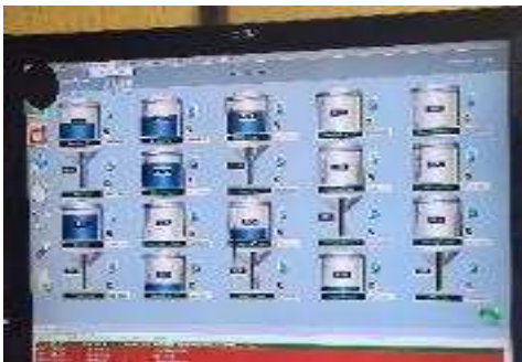
SCADA system at Balkfontein WTW
