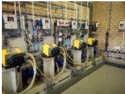
Ammonia dosing station
