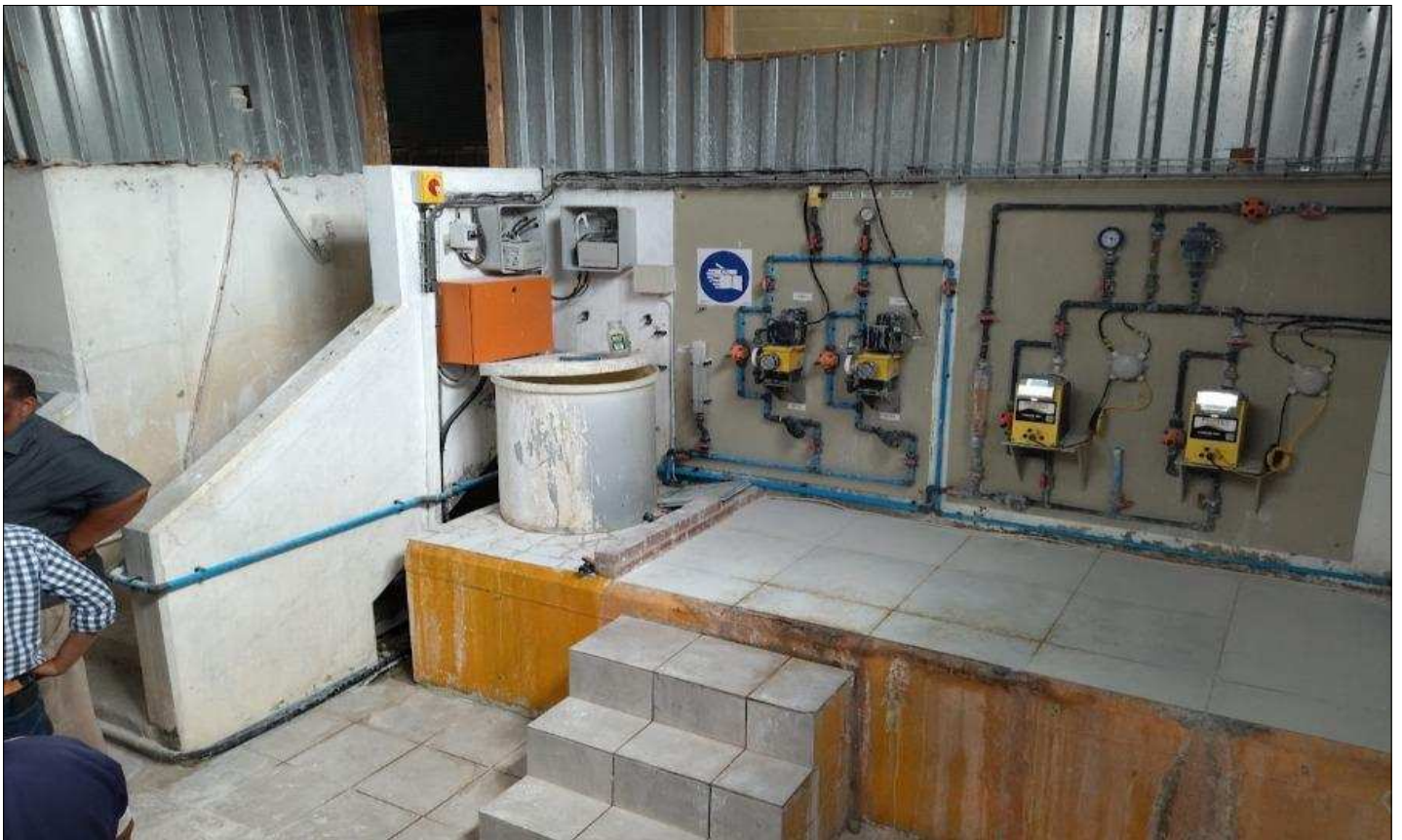
Grabouw WTW: Chemical dosing facility – accurate dosing and knowledgeable process controllers
