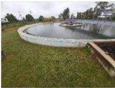
Sedimentation tank at Cullinan WTW
