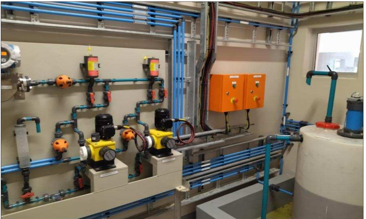
Drakenstein: Welvanpas WTW chemical dosing – textbook: a clean plant is a safe plant is a productive plant
