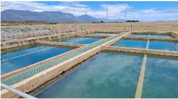
Sedimentation tank at Swartland WTP
