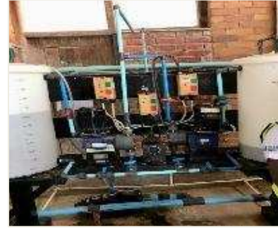
Chemical dosing units at both treatment plants with chemical dosing rates not verified
