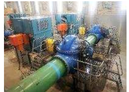
Distribution network pumps at Palmiet Pump Station
