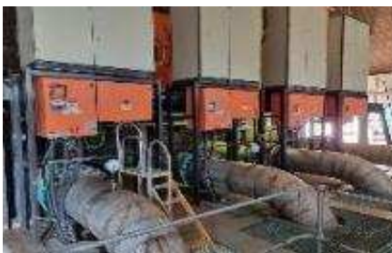
All pumps working - 4 installed 2 duty & 2 standby
