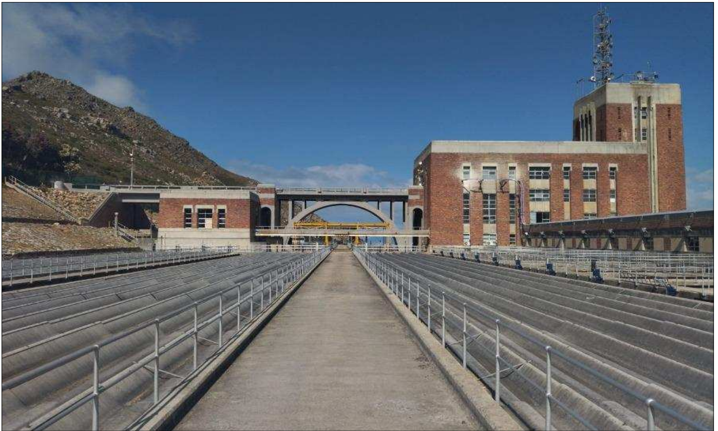
City of Cape Town, Steenbras WTW in pristine condition, well operated with competent staff
