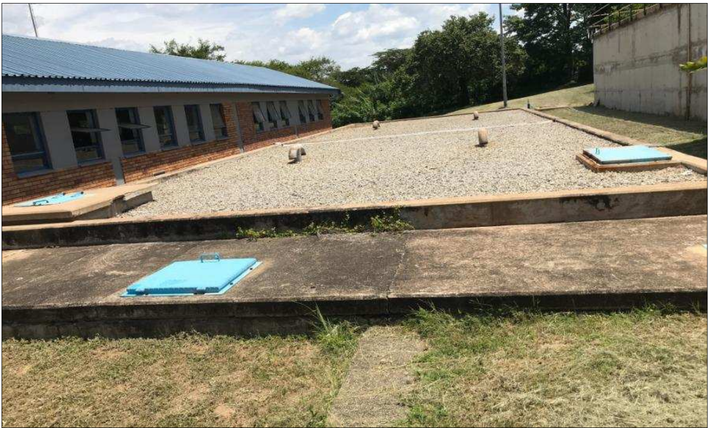
Mbombela: The new Nelspruit clear water tank is well maintained, proud housekeeping
