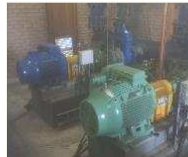
Pumps to the command reservoir
