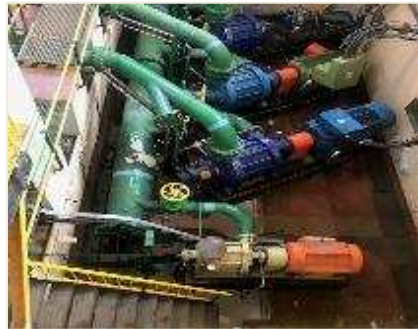
Final water pumps at both plants visited are in operational conditions
