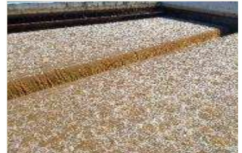
Backwashing cycle in progress
