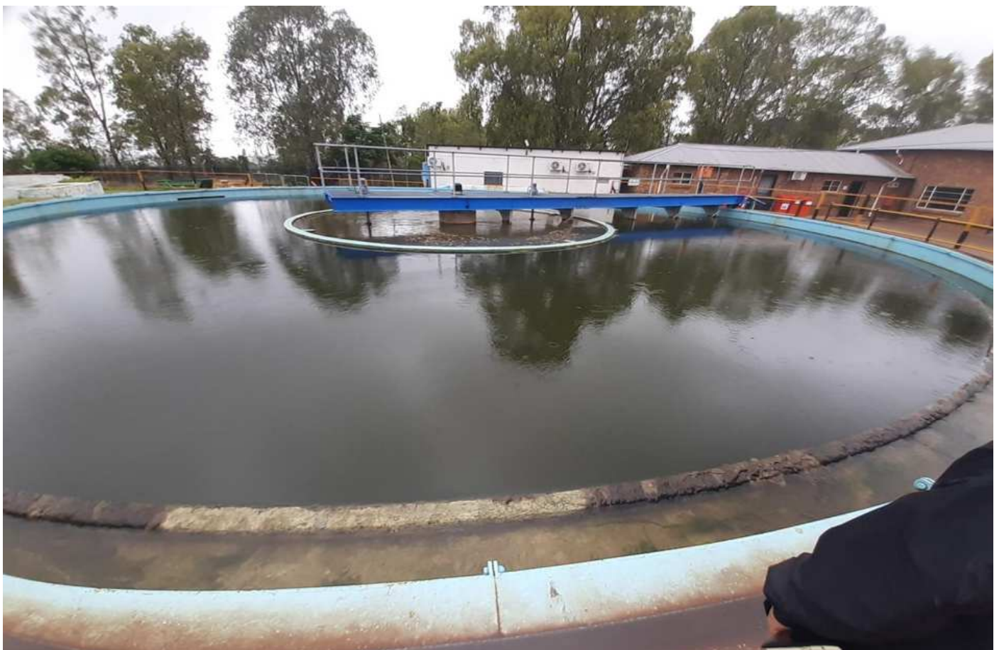
Clarification - essential to remove suspended solids to provide a clear, high quality potable water to consumers
