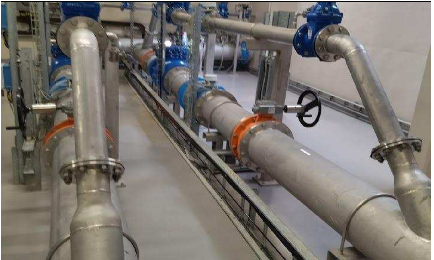
Drakenstein: Welvanpas raw water inlet work –clean, maintained, operated by a proud competent team
