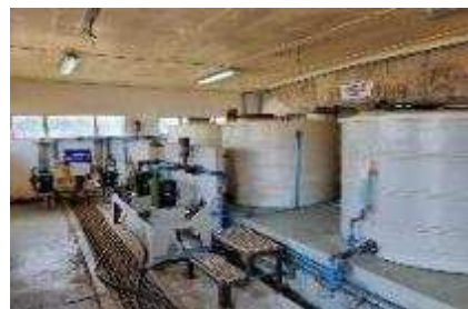
Chemical feed in a very good condition - duty/standby alum dosing noted dripping
