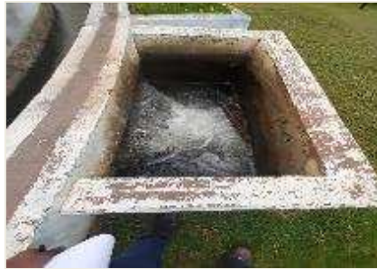
Overflow from sedimentation tanks
