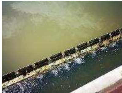
Clear overflow from sedimentation tanks
