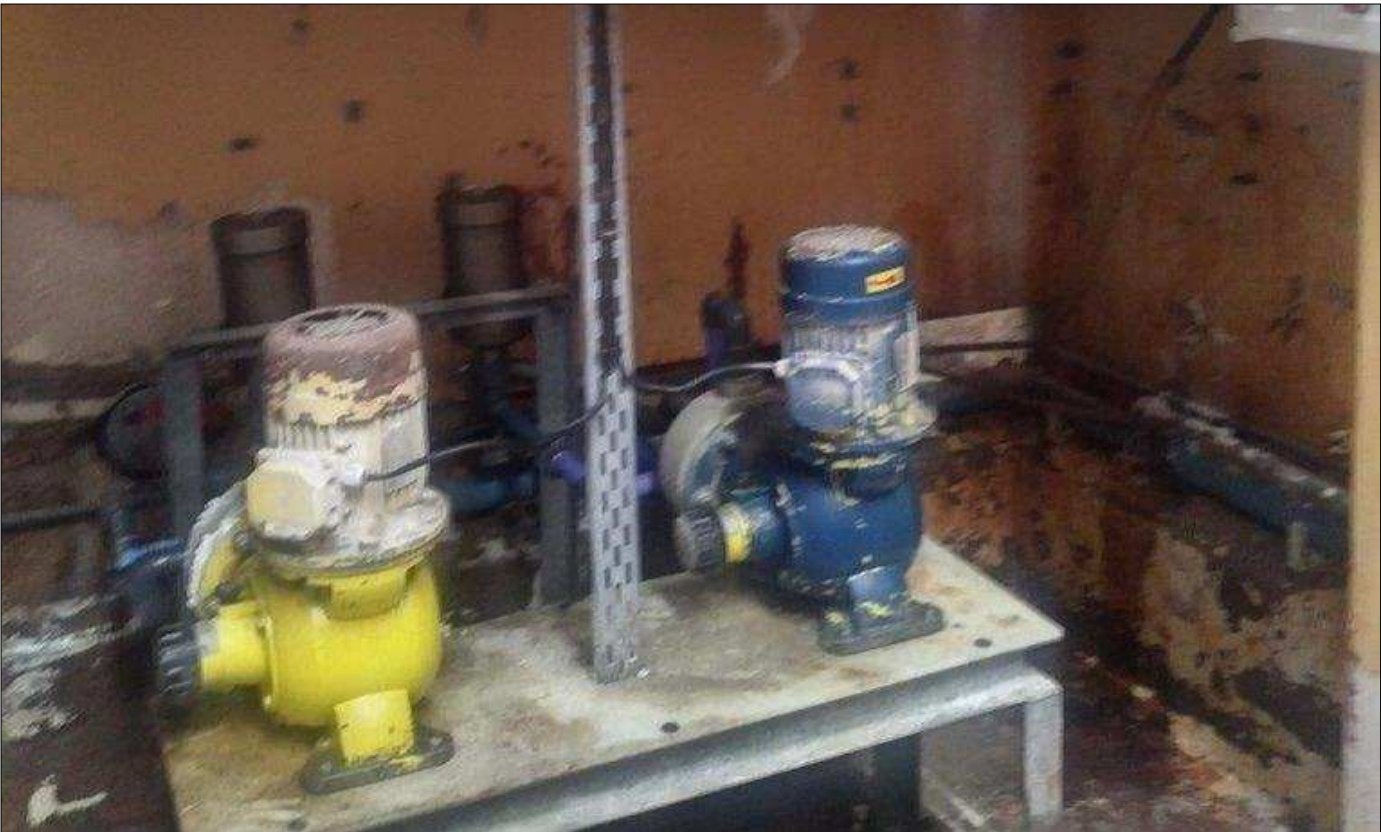
Chemical dosing pumps at the new George WTW
