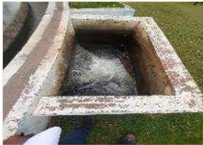
Overflow from sedimentation tanks
