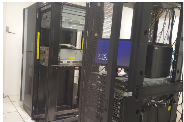
ICT Server Room Infrastructure
